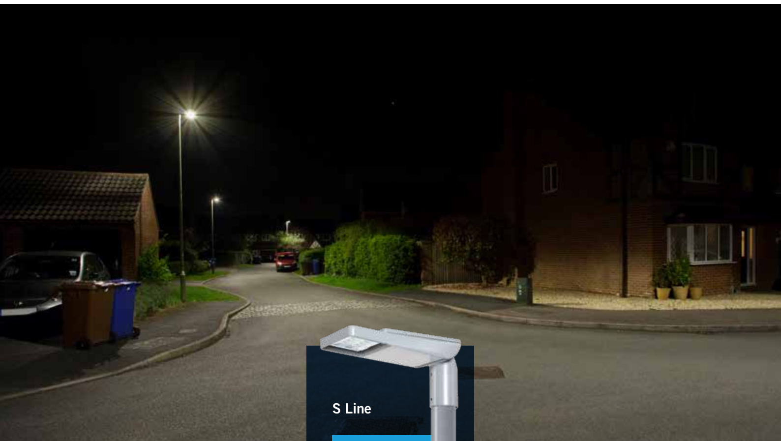
Previous 35W SOX installation
