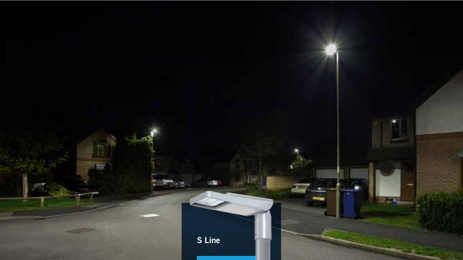
Previous 35W SOX installation
